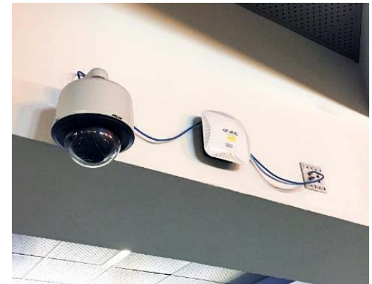
Photo taken at McCarran Airport in Las Vegas – Anyone could jump up and pull out the patch cord to the surveillance camera and wireless access point.
