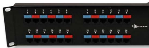
Patch Panel in a TR
