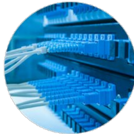
Opticalization: Datacenters Access networks Structured cabling
