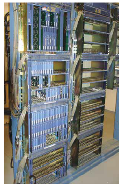
EXHIBIT 800.1 A private automatic branch exchange, which is one part of telecommunications equipment.
